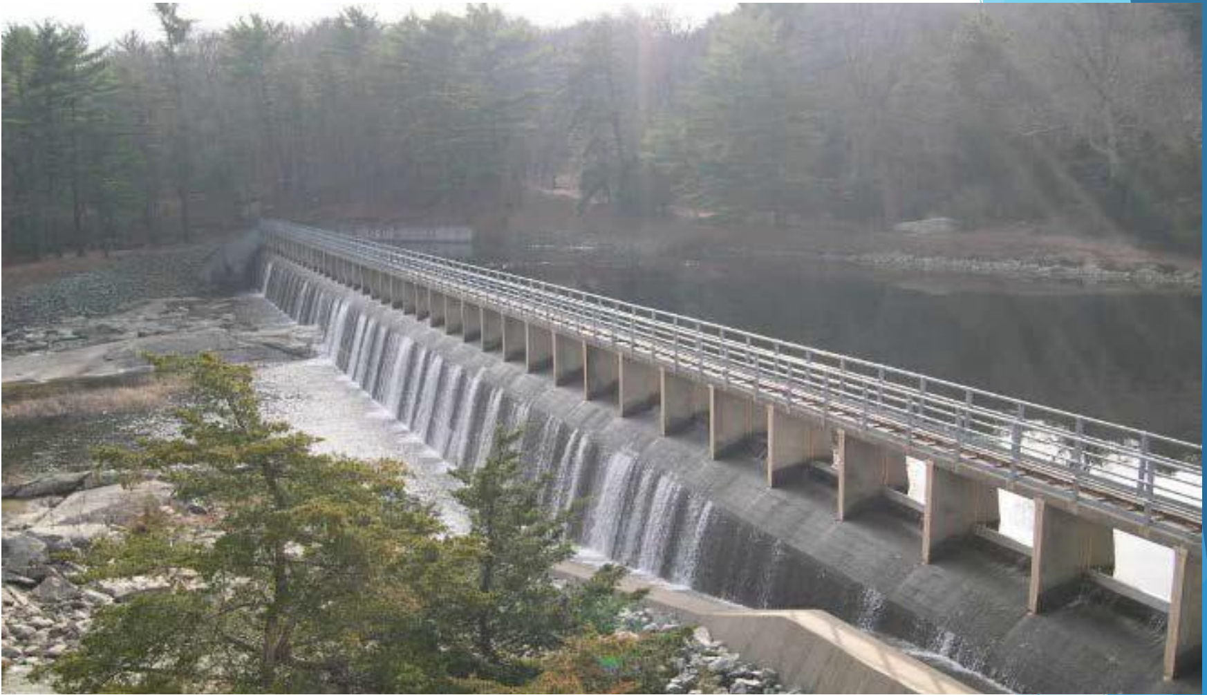
Figure 2: The Gainer Dam spillway on a normal day, with only a trickle being added to normal flows that come from the dam's central outlet, which feeds the North Branch of the Pawtuxet River. See Figure 3 for an image of the spillway's raging torrent on March 31st, 2010. National Weather Service Northeast River Forecast Center (NWS/NERFC)
